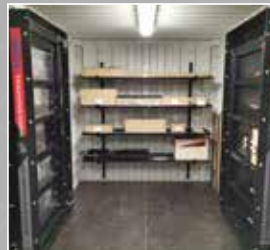
Storage for spare parts
